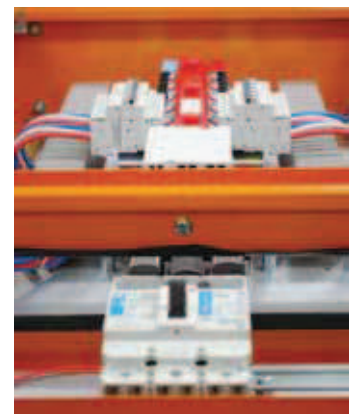
Several main switch options including 250A MCCB Mainswitch for cascading up to 30kA using 6kA outgoers
