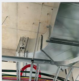
Mechanical HVAC, Pipe & Ductwork
