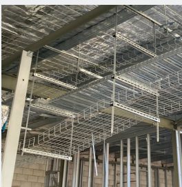
Electrical Services & Cable Tray
